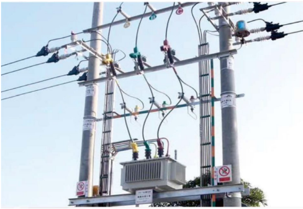
Overhead line courts
